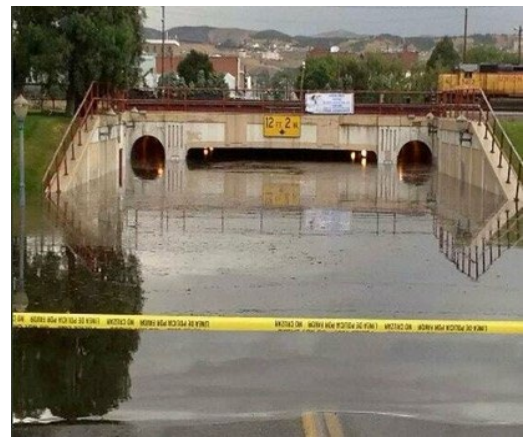
Figure 21 Flooding of the Center Street Underpass in Pocatello
