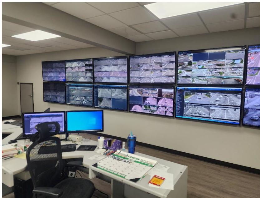
Figure 11 The City Pocatello Traffic Operation Center
